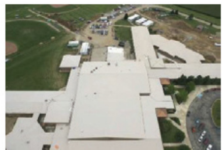
Finding a roof that could not only last for a long time but look good and match the existing metal was a challenge for West Liberty High School. Duro-Fleece 60-mil membrane provided both and proved the right choice for the job.
