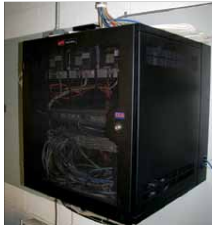
CyberLock Installed in a Net Shelter Box (Photo provided by Robert Blickensdorf at ITC)
