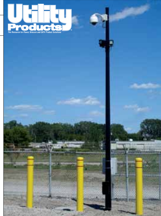
Live camera mounted on a pole by perimeter fence. (Photo provided by Robert Blickensdorf at ITC)
