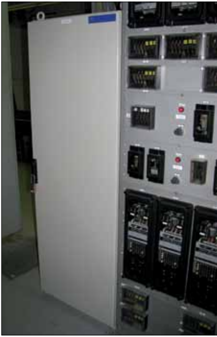
CyberLock Padlock on an ITU Cabinet (Photo provided by Robert Blickensdorf at ITC)
